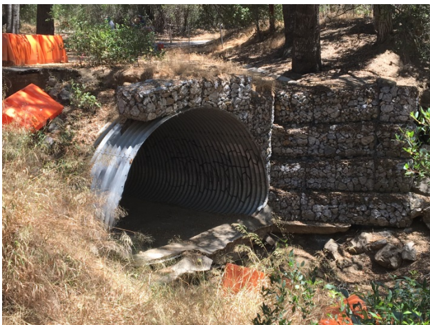
Existing culvert with washed out gabions
